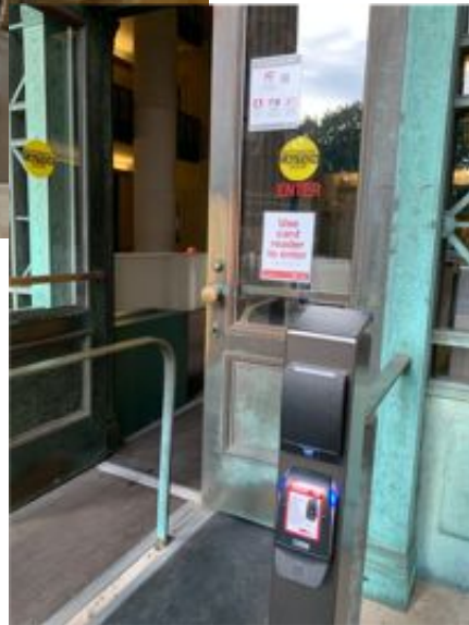
ID and QR Readers installed at exterior doors
